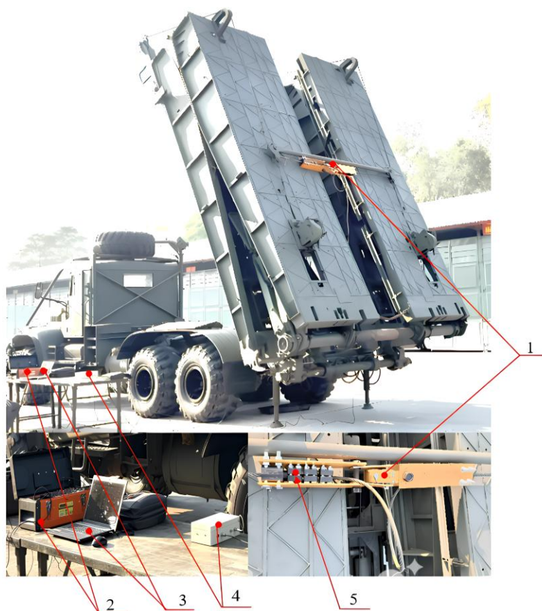
Figure 4. On-site experimental setup for measuring cable tension: 1- LCMGD sensor; 2- Ni-6009; 3- Computer; 4- Amplifier; 5- Fixture for converting tensile force to compressive force.
