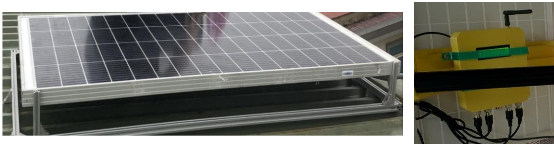
Figure 9. Experimental deployment of data acquisition and monitoring for the PV system.
