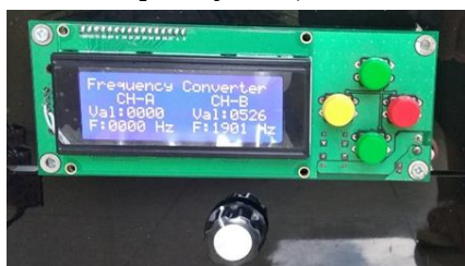
Figure 2. The layout of equipment TR-1 used to change the physicochemical properties of wastewater.
